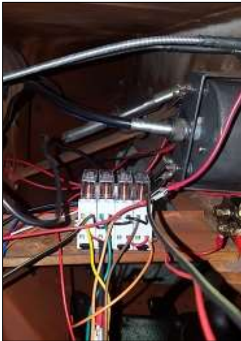
Figure 8: Relays bolted to top of support bracket underneath the cowl
