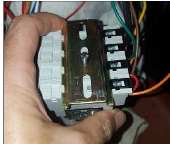
Figure 6: Relays loaded onto DIN rail
