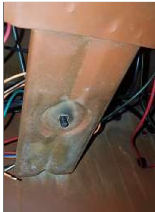
Figure 7: Dash to firewall support bracket, with 1/4" bolt for securing DIN rail and relays
